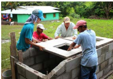
Construction of an improved cookstove by Toño, Chico, Pablo, and Panfilo in El Espino, Nicaragua. Photo taken in 2013 by Becky Miller, a Green Empowerment intern.
