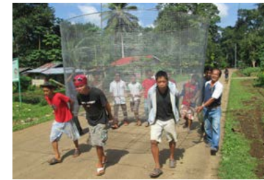
Community volunteers haul rebar for the reservoir tank of their ram pump water system. Photo taken in 2013 in Mampalam, Talipao, Sulu, Philippines.
