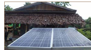
New solar installation at the Free Burma Ranger office in Dooplaya District, Karen State, Myanmar. Photo taken in July 2014.
