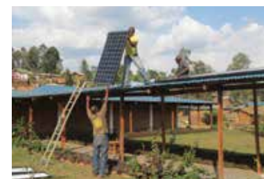
Solar power installation at The City of Joy, 2012.
