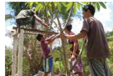
Solar power installation in Thaninthary Division, Myanmar, 2012.
